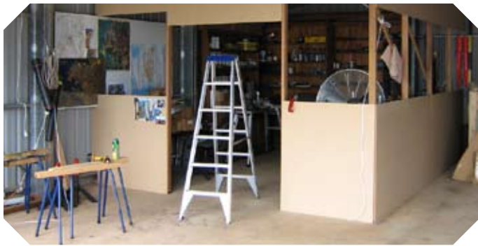
Paul's first task was to build a cool room in his hanger. "It's a prerequisite for building in Darwin!"
